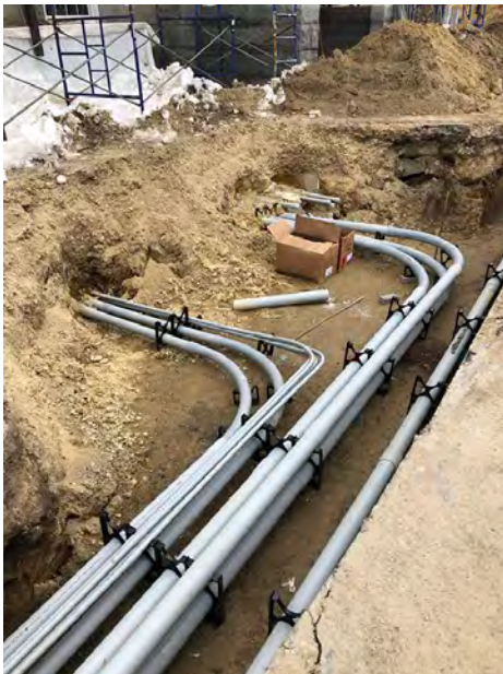
Conduit Feeds into Building from Transformer and Emergency Generator to Electrical Room
