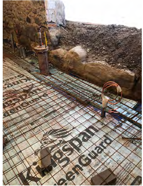
Water Piping for Fire Suppression System and Domestic Water Supply System
