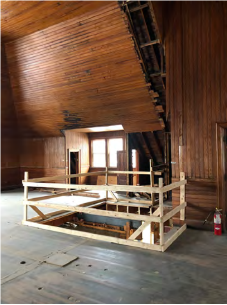
Third Floor Guardrails and Toe Kick Boards at Elevator Hoistway Opening
