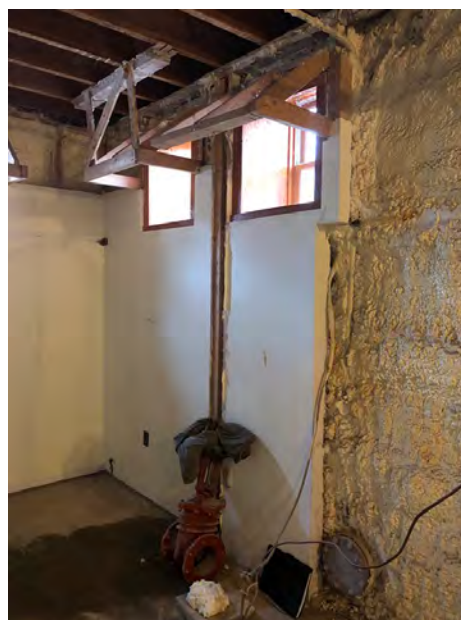
Former Window Wells at Northwest Corner of Community Education Office
