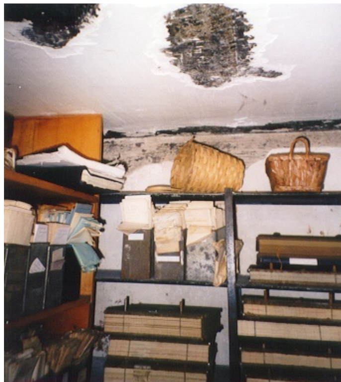
Portions of the ceiling are falling; the binders have hinges that are rusting due to the excessive dampness.
