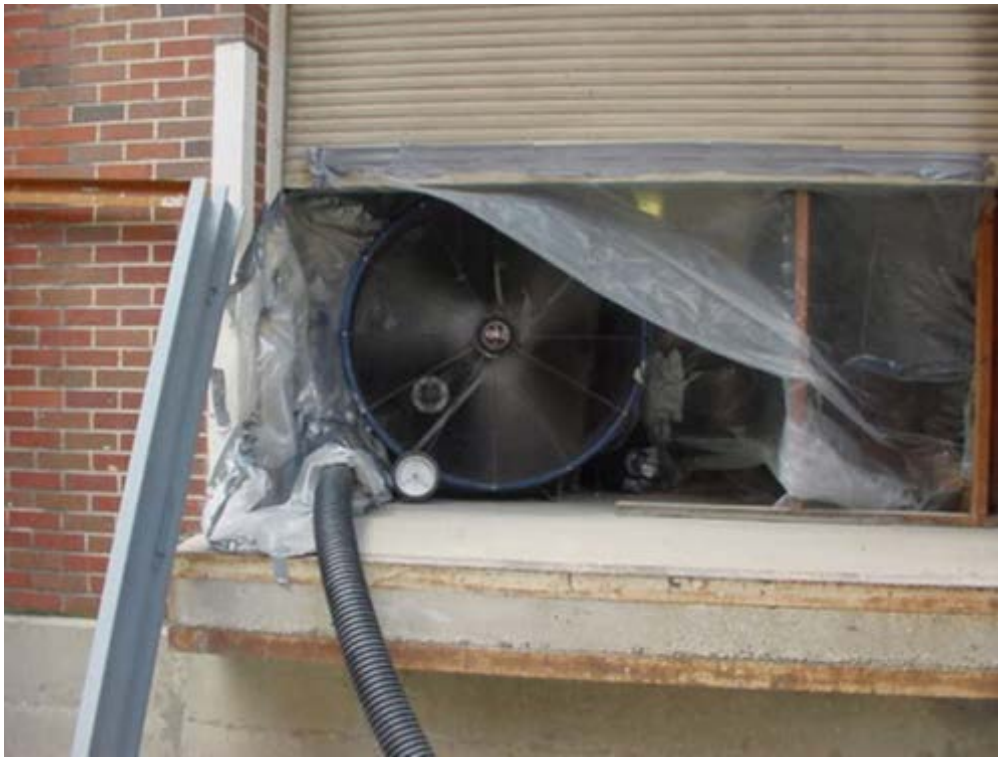
Photograph 9-6 View of ventilation with an industrial fan
