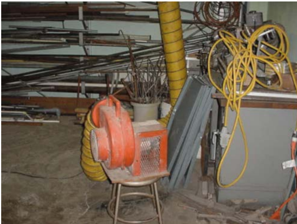
Photograph 9-7 View of ventilation with a blower unit
